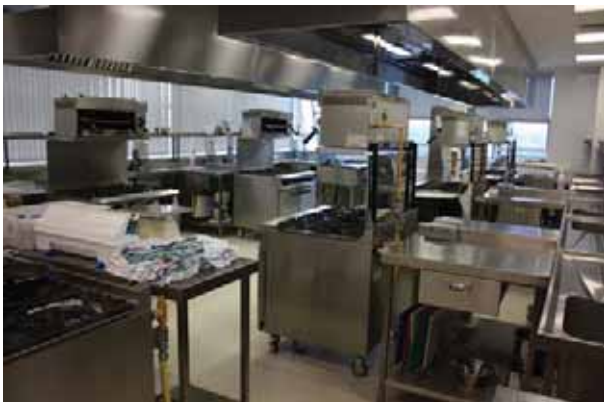
Catering production kitchen South Lanarkshire College (photo: AMA)
